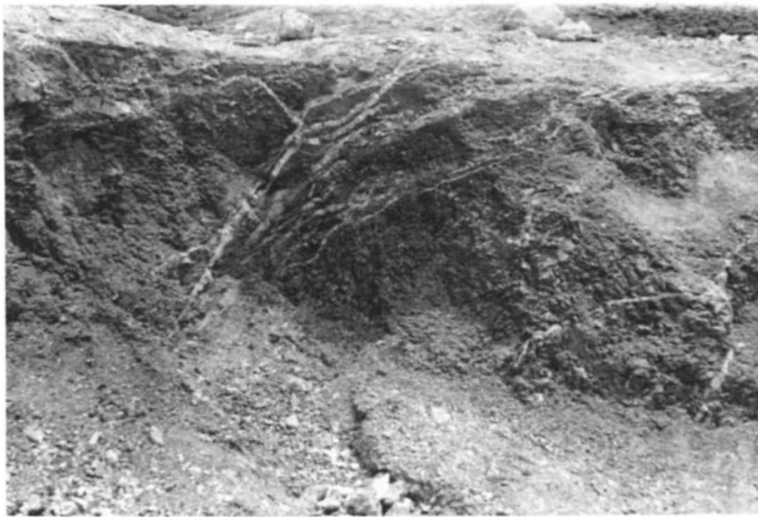
Fig. 4.9 Fissure filled with clay/cement grout in the excavation for the Peruča Dam foundation
