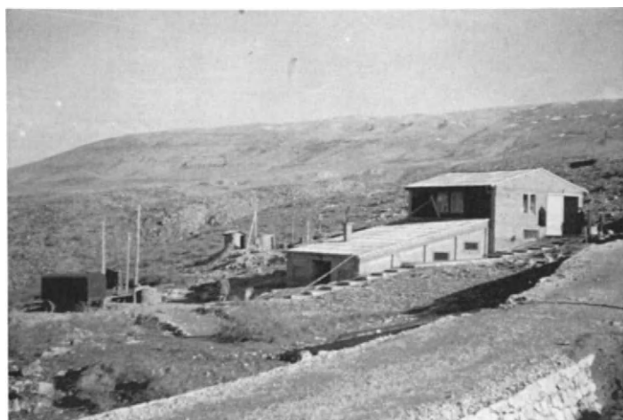
Fig. 5.17 View of the grouting plant for the Peruča Dam
