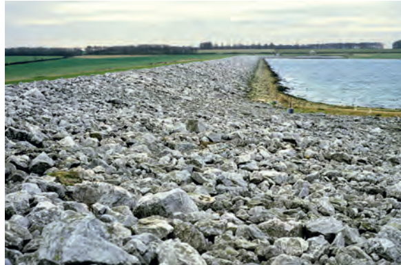
Limestone rip-rap prevents erosion on a reservoir, but is expensively carried 90 km to site by road.
