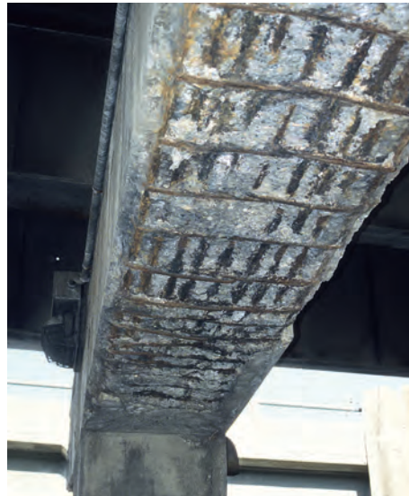
A concrete beam supporting a freeway, with its reinforcing bars exposed by spalling after corrosion of the steel in a concrete mixed with salty water.
