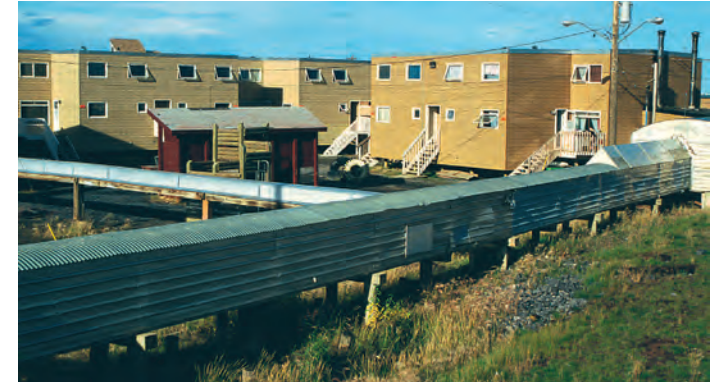
Linking houses elevated on piles, utilidors carry inbound water and outbound waste inside insulated tunnels perched on timber piles, to eliminate heat losses into the permafrost.
