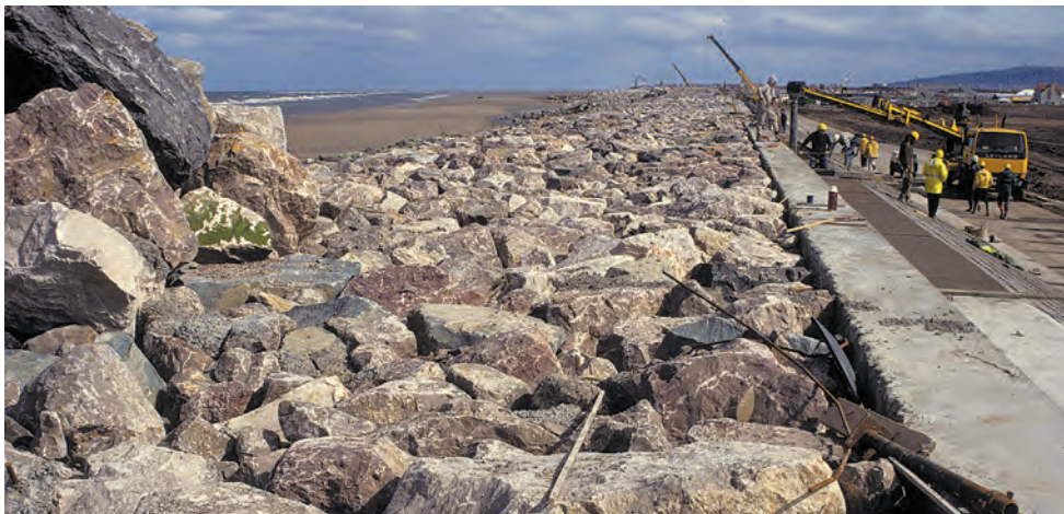
At Towyn, sea defences have 4-tonne blocks of limestone placed individually by a grab.
