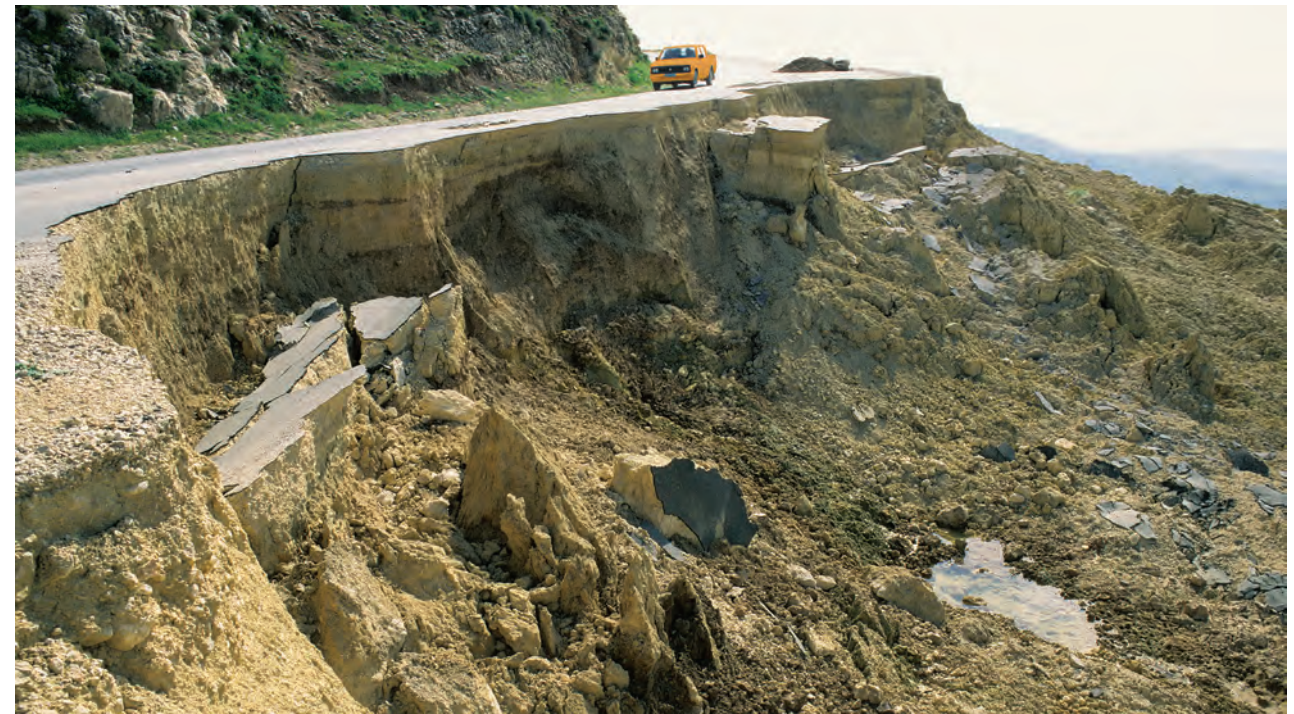
A road undermined by multiple failures of hillside soils and artificial fill after a heavy rain storm event.
