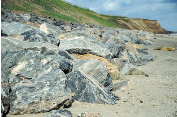
Armour stone of 5-tonne blocks of strong gneiss, economically carried 700 km to site by sea.
