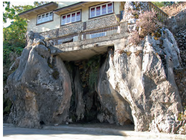
A building placed on a reinforced concrete slab that is supported entirely on adjacent pinnacles of strong limestone in karst of class kIV, spanning a void that was filled with clay and is now exposed in the hillside.
