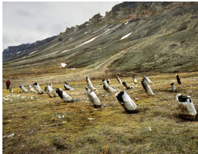
Timber piles that were placed through the active layer and founded in permanently frozen stable ground; the wooden building on them was then burned down, since when 50 years of solifluction and creep of the hillside soils have rotated the piles above their stable toes.
