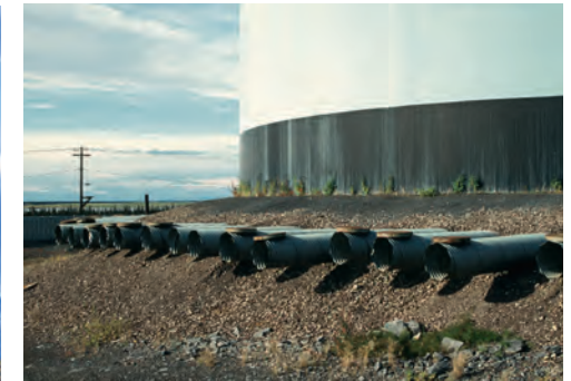
Steel ducts carry cold winter air through a gravel pad to conserve the permafrost beneath a large, warm storage tank.
