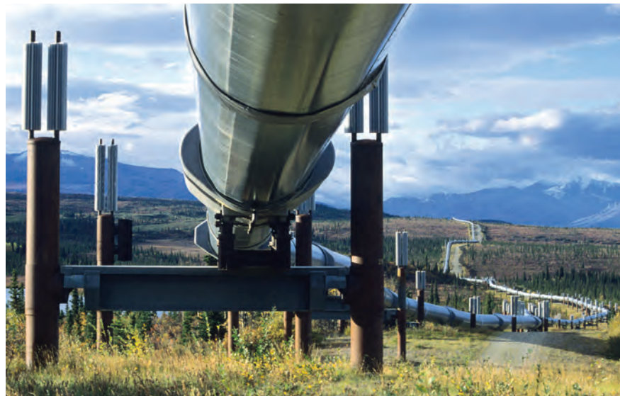
Carrying warm oil, the Trans-Alaska Pipeline is supported on trestles with piles into the frozen ground beneath the active layer; each pile has internal ammonia refrigeration with rising gas and sinking liquid that transfers heat from the ground to radiator fins above, and thereby conserves the permafrost.
