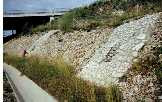
Road cutting with breached caves that have been closed by masonry except for access openings; the road was built on an impermeable base to avoid disturbing ground drainage.
