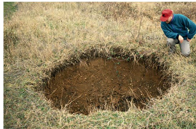
A new subsidence sinkhole in soil that overlies chalk, formed immediately after a water main had burst nearby.
