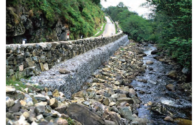
A road has to lie along a river bank in a narrow valley, so has a gabion wall to prevent fluvial erosion undermining it during predictable high flood flows.
