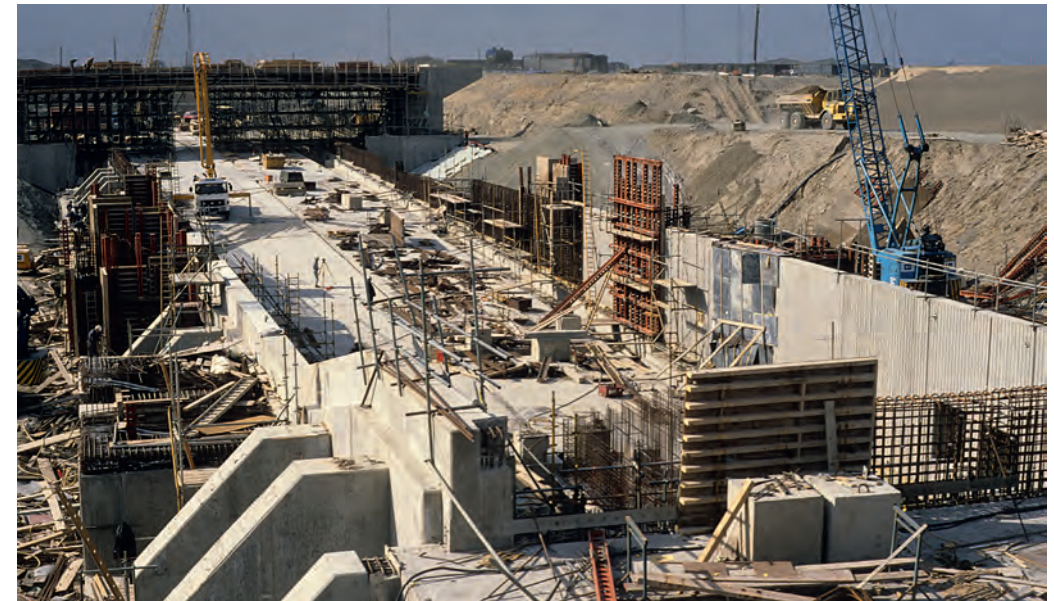
The tunnel under the River Conway is a submerged tube that has approaches in deep cuttings with retaining walls; a thickened concrete base was made with a dense aggregate to hold the structure down and prevent it floating upwards where it lies beneath the water table.
