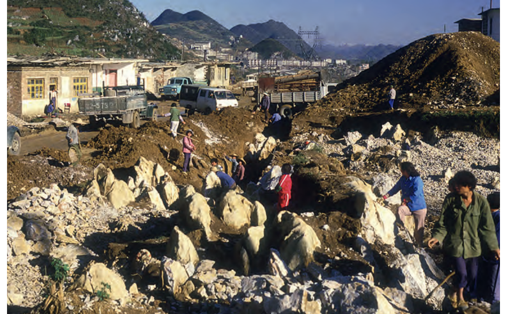
Limestone pinnacles exposed on a building site in class kIV karst, before digging out the clay soil, breaking off the pinnacle tops and filling the fissures with broken rock.
