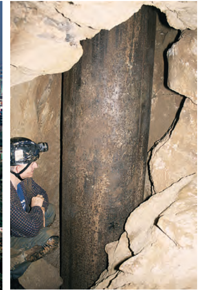
The casing of a bored pile that was constructed through a cave to reach footing on intact limestone beneath.
