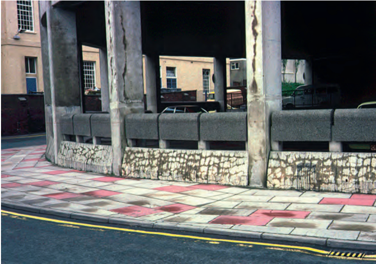
Concrete with deep cracks due to alkali-silica reactivity in marine aggregate, in the wall and columns of a multi-storey car park.
