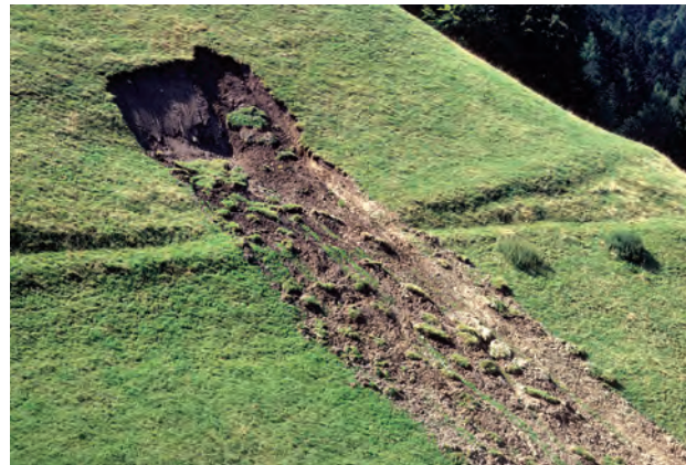
A shallow landslide that is just one consequence of long-term weathering of a hillside creating a soil that becomes progressively thicker and weaker until it fails, typically when saturated by a heavy rainfall event
