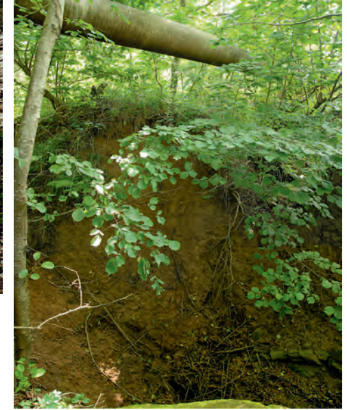
[above right] Pipeline that has been left suspended over a new sinkhole, which formed in the soil cover where the drainage had been disturbed by excavation of the pipeline trench.
