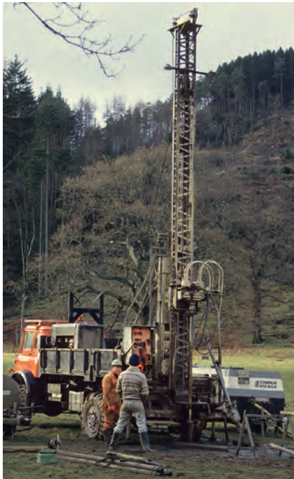
[below left] A truck-mounted hydraulic drill at a ground investigation, coring bedrock beneath a few metres of cased hole through overburden.
