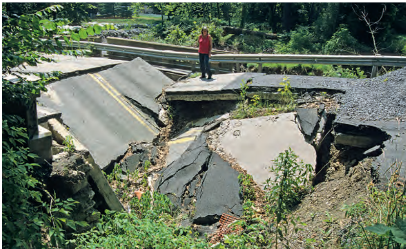
Road destroyed by a new sinkhole where the underlying soil was lost into karst limestone of class kIII when inflow and suffusion were increased by water-table decline due to pumped drainage of a nearby quarry.
