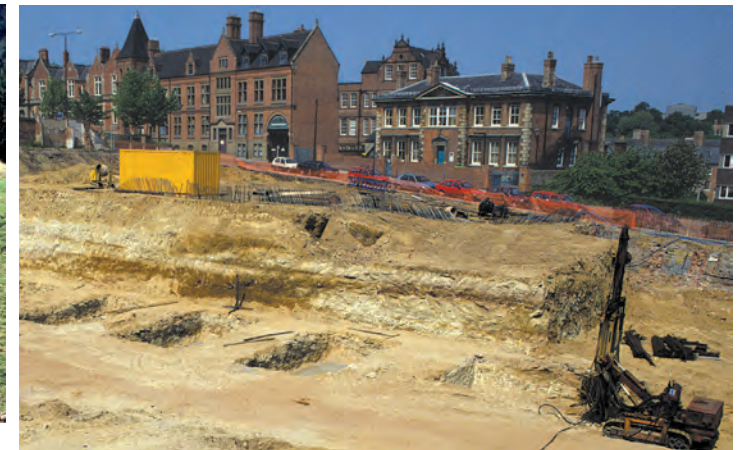
Weathered sandstone exposed on a building site; the upper three metres have been removed so that the concrete column bases can be cast in less-weathered, stronger rock beneath.
