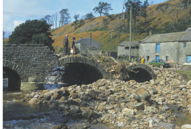
An old stone bridge that was largely destroyed when it was overtopped by a short-lived flood flow that was too large to pass through its arches.
