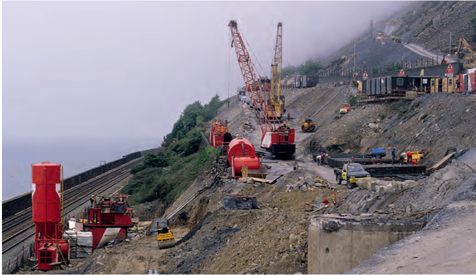
Early excavation work shows the very constricted site, with the live railway below.
