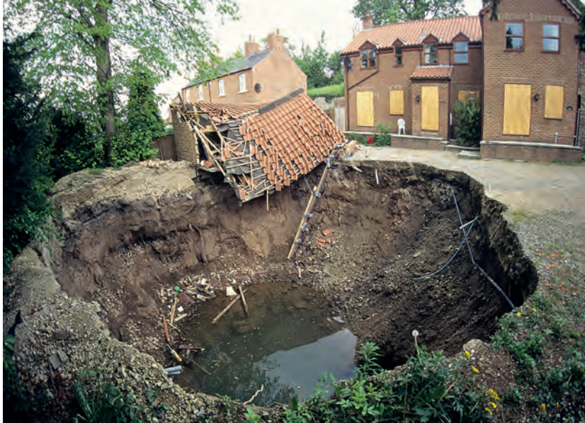
Catastrophic sinkhole collapse in gypsum karst, at a site undermined by a breccia pipe forming in the gypsum beneath 15 metres of soil cover.
