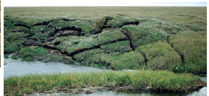
Ground subsidence over large ice wedges thawed when invaded by warm summer drainage water from a road.
