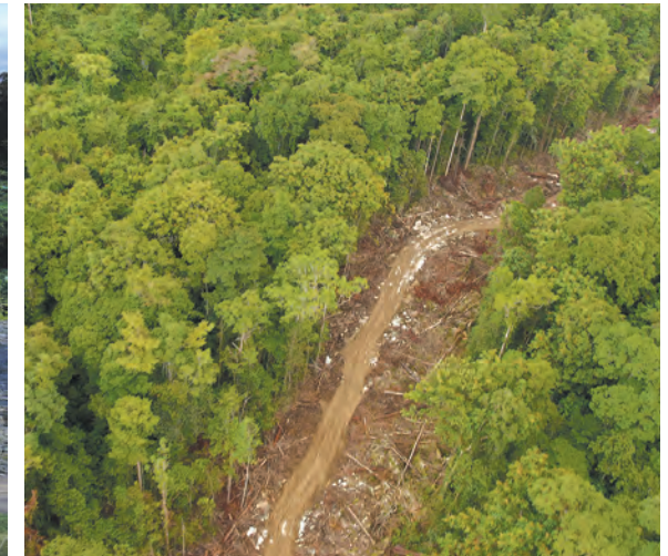
The density of equatorial rain forest precludes detailed prior ground investigation for any road or pipeline driven through it, and the necessary tree clearance turns the site into a mudbath.
