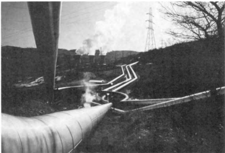
FIG. 4.15. Steam pipeline feeding Larderello 3 at Casuonova power plant.
