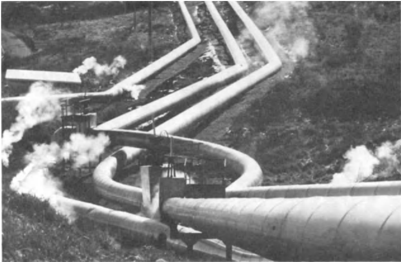
FIG. 4.16. Steam pipeline feeding Larderello 3 at Casuonova power plant.
