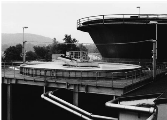
Fig. 12.4. 55 ft-diameter DAF clarifier.
