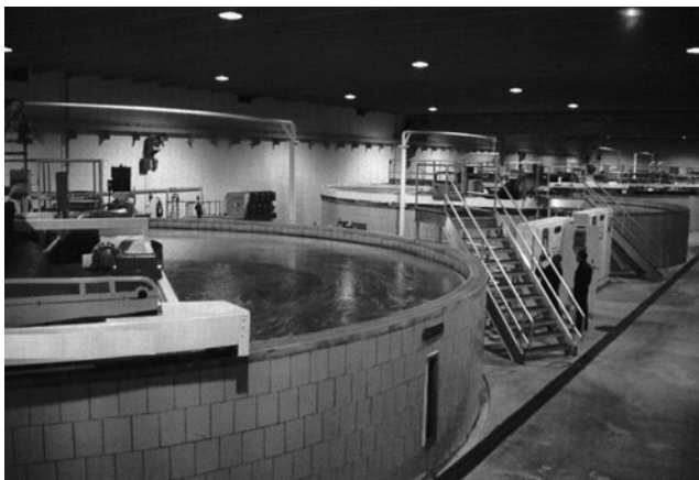
Fig. 15.4. Flotation–filtration clarifiers at Cleveland plant.
