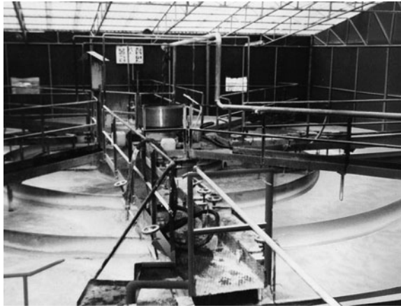
Fig. 12.2. An installation with a 40 ft-diameter IAF cell.
