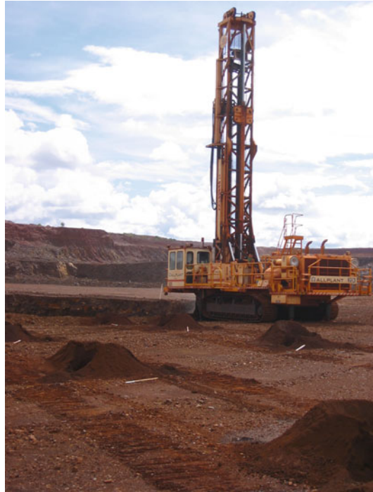
Fig. 4.21 Drilling blastholes using truck mounted open hole percussion drill rig, Yandi iron-ore mine, Western Australia
